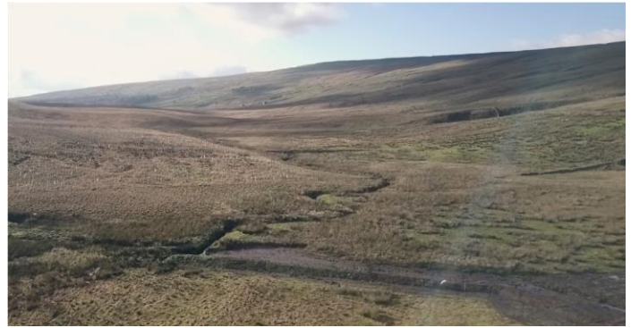
One of the Low Level Earth Bunds from the sky installed at Swarthghyll Farm on Oughtershaw Beck.
